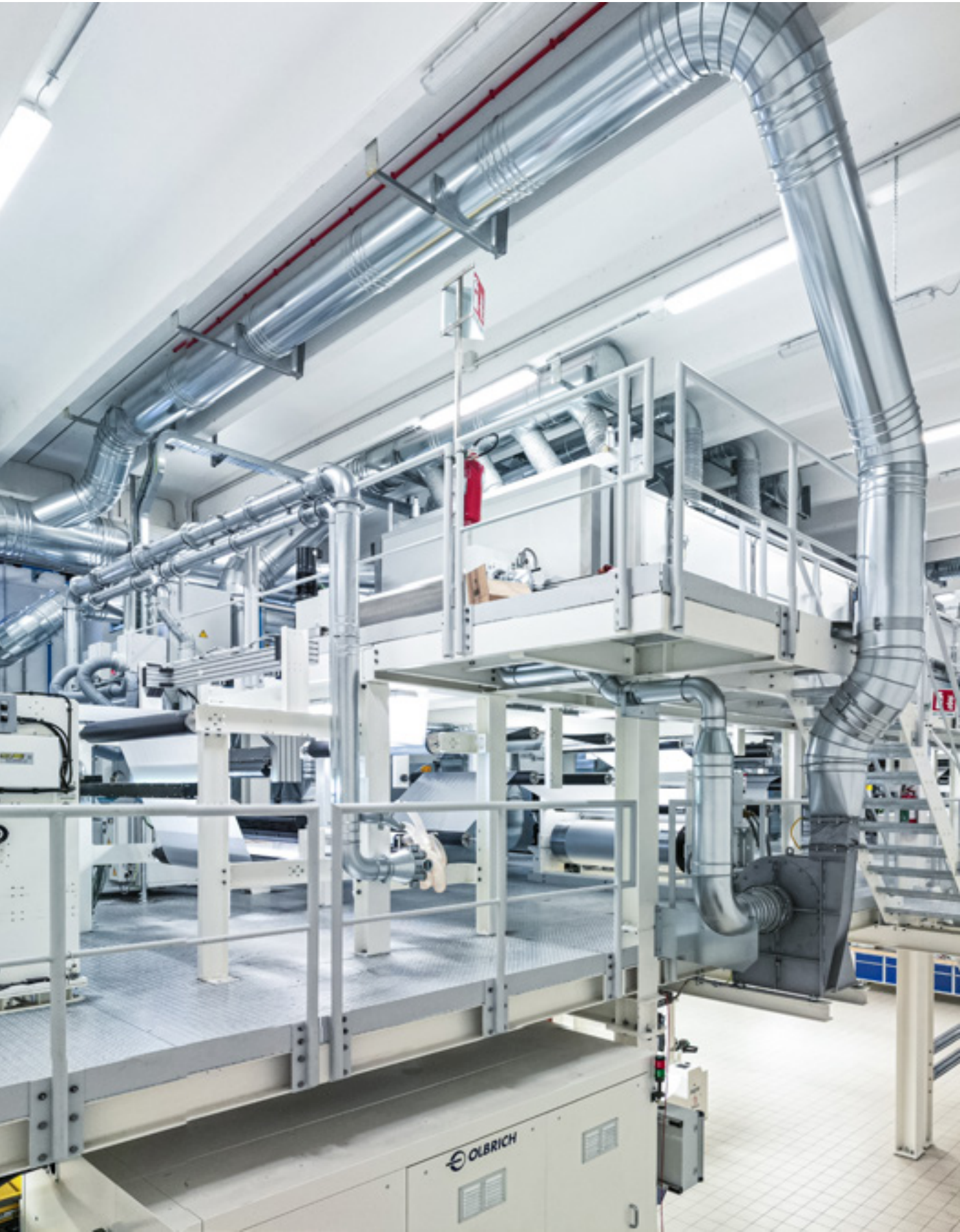
Film coating and heat-stabilisation production line
